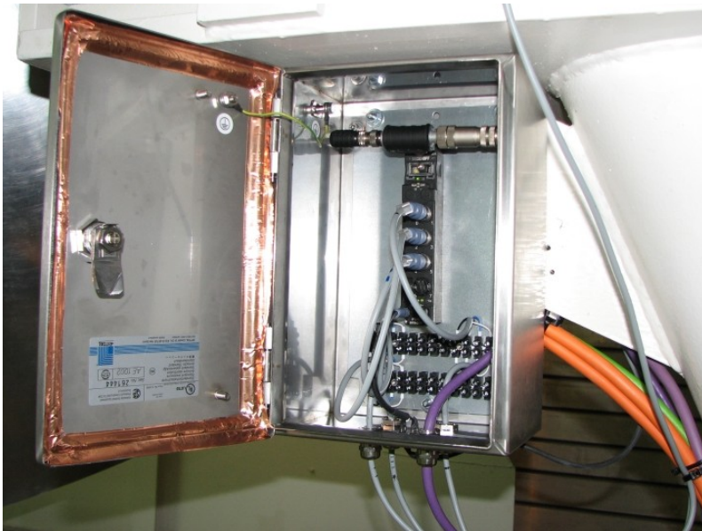
M3 Mirror Profibus Module inside shielded box
